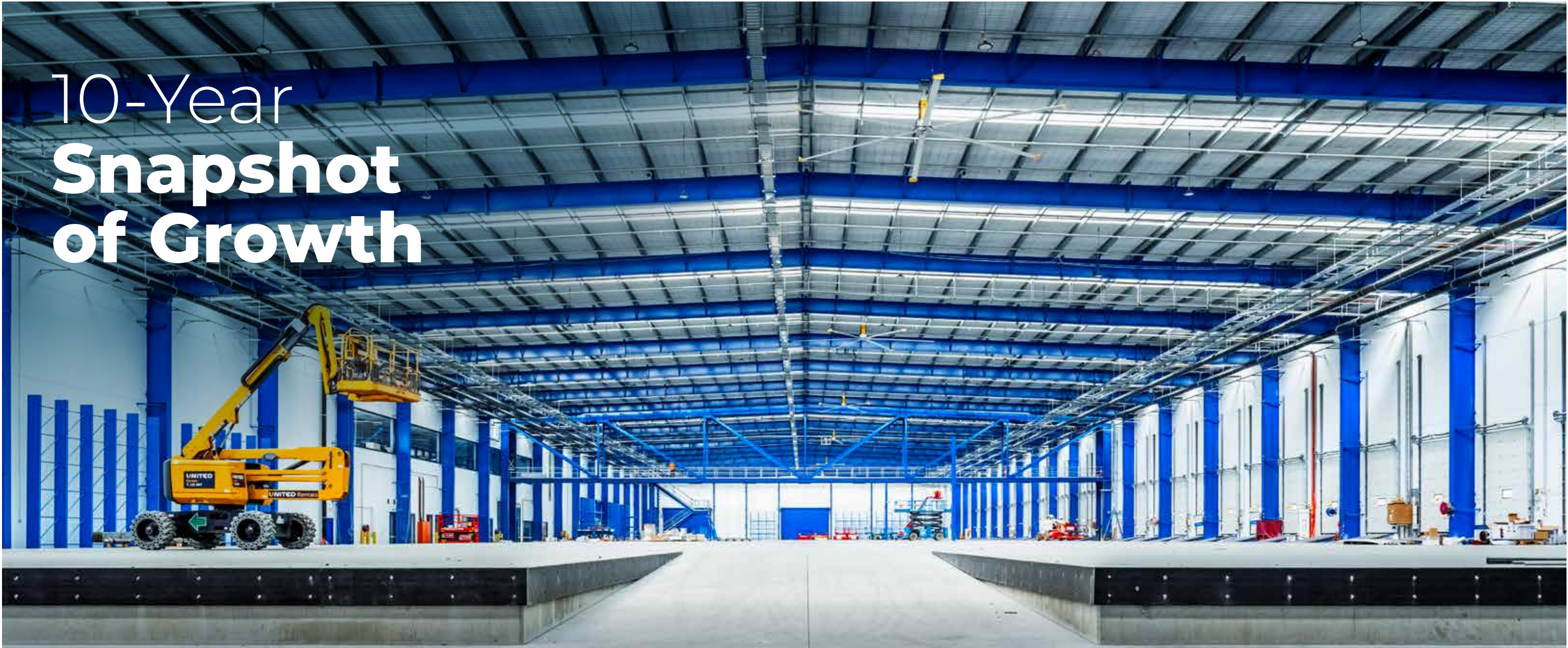
OUR NEW 15,298 M 2 CROSSDOCK FACILITY WITH 34 REAR-LOADING DOORS. UNDER CONSTRUCTION AND DUE TO OPEN JUNE 2026. WILLAWONG, BRISBANE, AUSTRALIA
